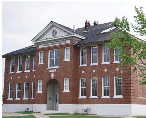
Sheridan School District’s Admin Building, built in 1913, still operational today, and required special attention during district-wide roofing project
